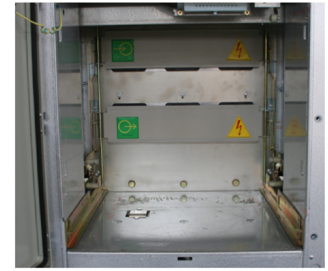
In the separate room of the circuit breaker, open the metal valve to check the static contact.
