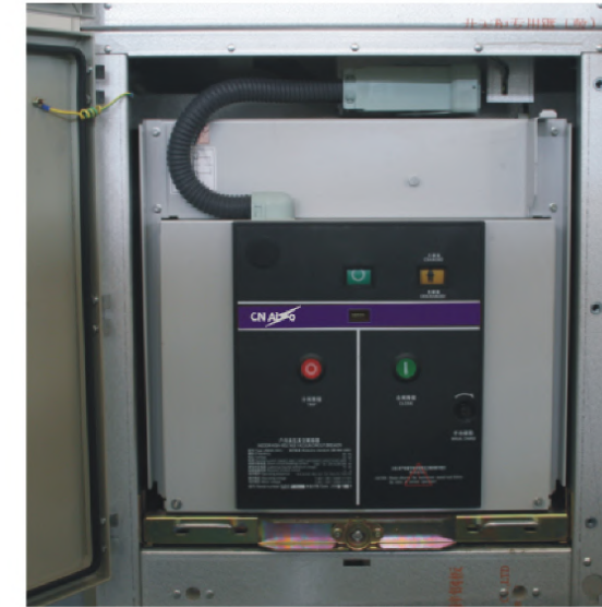
Draw-out circuit breaker room
